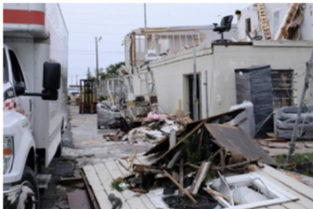
Gaige Davila, "Destruction of homes—most of which were not up to code—in colonia Laguna Heights following a tornado," Texas Public Radio, United States 12
